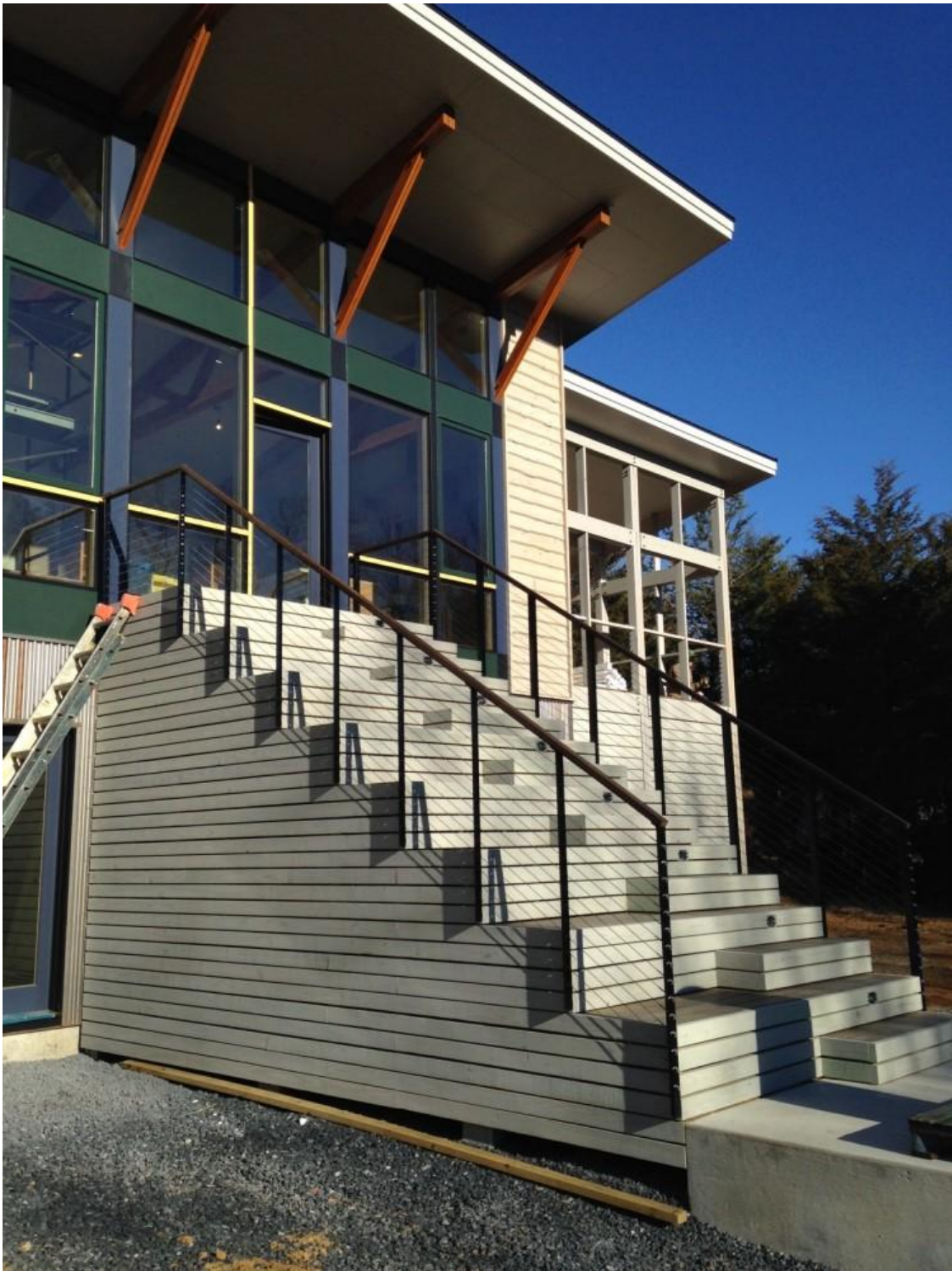
The monumental staircase that also serves as a sitting and outside entertaining space.
